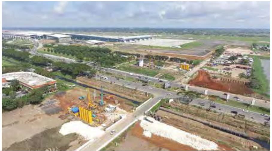
To meet the increasing number of flights and to optimise the time taken for ground handling of individual aircraft, the Soekarno-Hatta International Airport is building a new taxiway to connect the existing runways at the east side of the airport.
