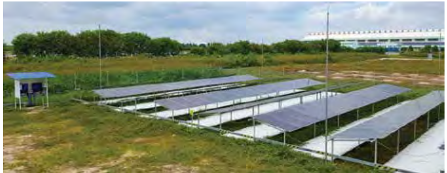
Completed in October 2018, the EDF's microgrid on Semakau Island will serve as a test bed for renewable energy that combines solar photovoltaic (PV) panels, wind turbines, and other new sophisticated technologies.
