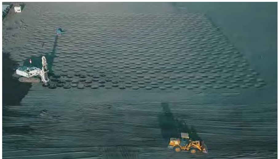
ABOVE: The Vantage-RIC method on the NYIA project involved hydraulically dropping a 9 t hammer from a controlled height onto a steel plate (compactor foot). The plate remains in constant contact with the ground, thus ensuring an efficient and safe transfer of energy.
