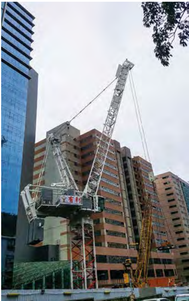
A Potain MR 618 tower crane helps to build a new private hospital in downtown Hong Kong.
