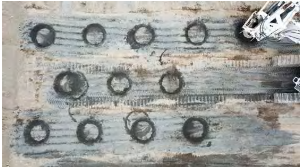
Vantage geotechnical engineers design a compaction pattern in advance, based on the geotechnical analysis carried out prior to the compaction work. Each individual compaction point is shown on a distribution plan and this is subsequently transferred into the on-board computer. With the sensor readings, the company is able to optimise the grid and in turn save time and resources.
