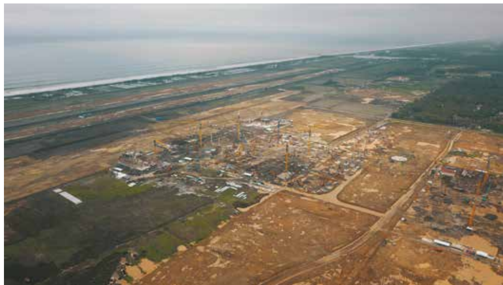
BELOW: Once completed, NYIA will replace the existing Adisutjipto International Airport. The new airport is said to be the first project in Indonesia that has adopted a fully GPS-guided and sensor-controlled RIC technology for ground improvement.
