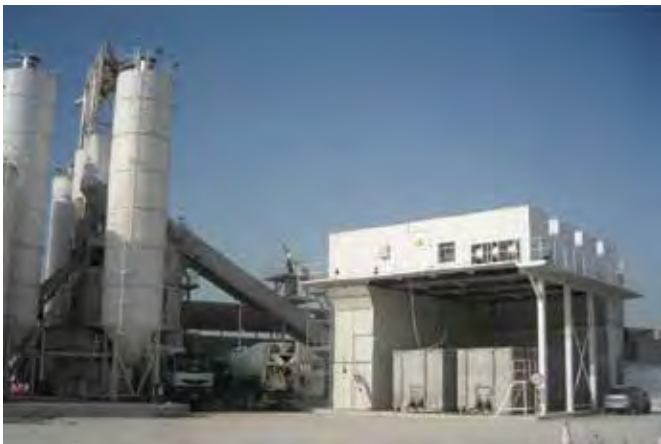
Lintec LEA100 concrete cooling ice plant and storage container arrangement for a maximum production capacity of 400 t /day.
